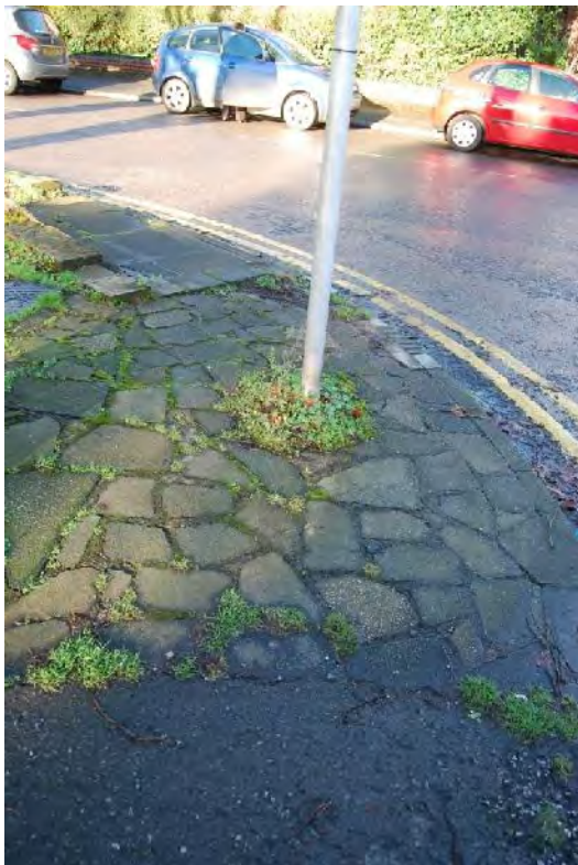
Uneven pavement at The Green
