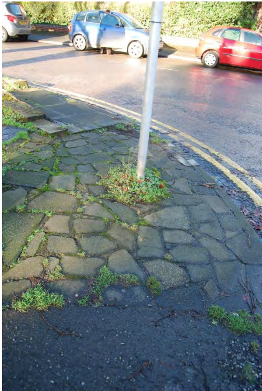
Uneven pavement at The Green
